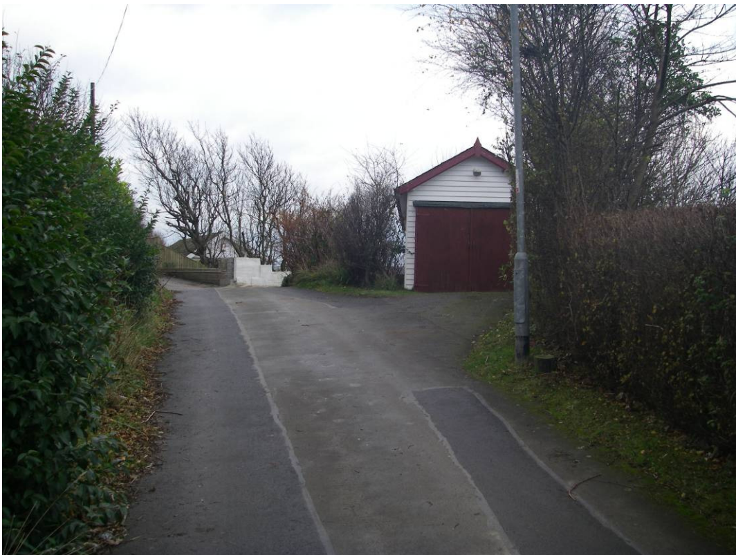
Plate 56 Site view of leaning timber garage at No. 5 Flat Cliffs, seaward of coastal slopes.
