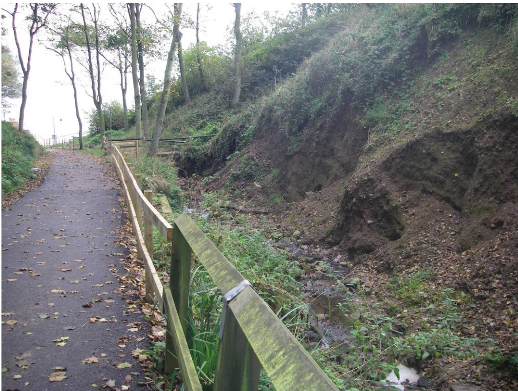
Plate 46 Site view of slope failures towards the base of Martin's Ravine.
