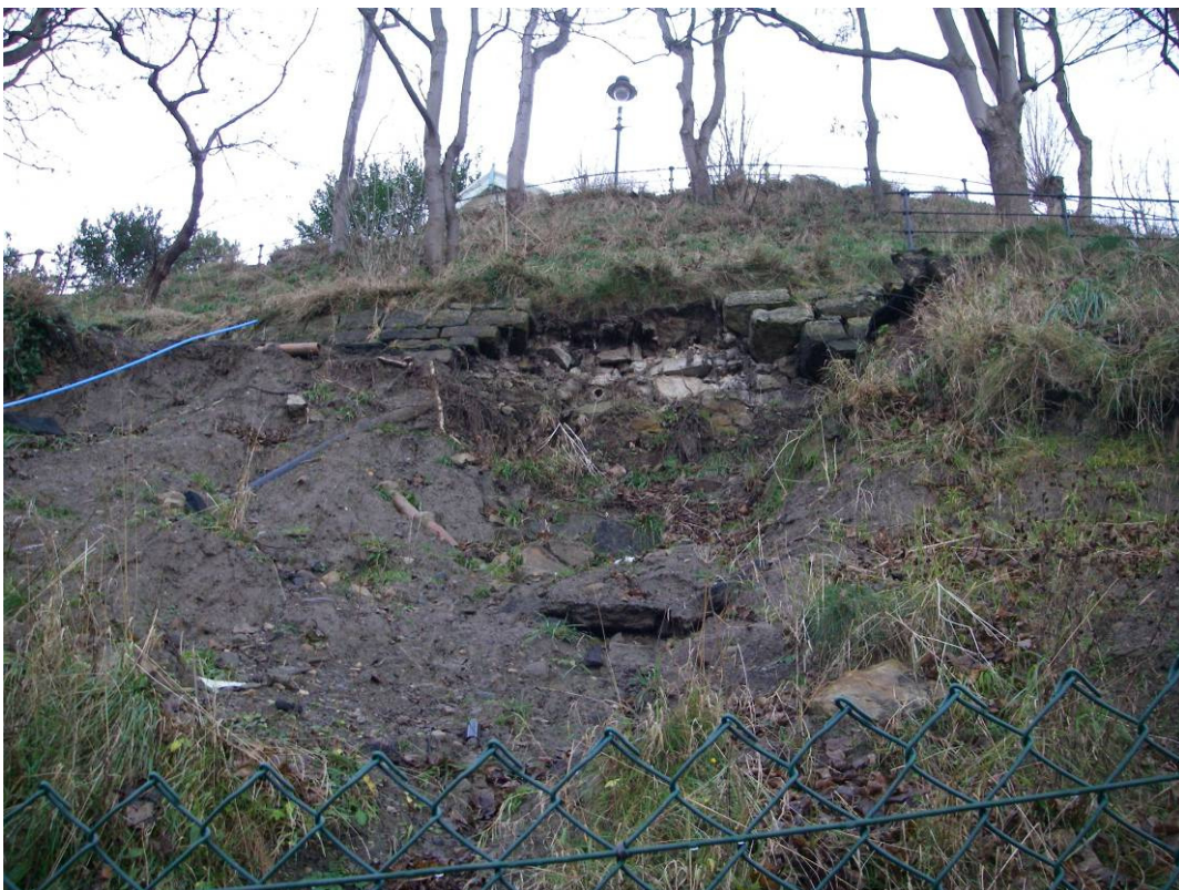
Plate 30 Site view of retaining wall and slope failure behind The Spa on Spa Cliff.
