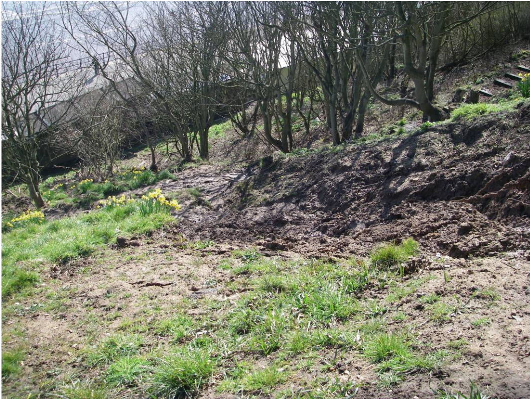
Plate 43. Site view from Glen Gardens looking down slope failure to Royal Parade.
