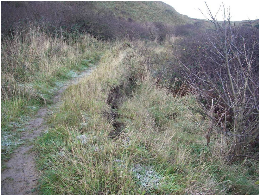
Plate 14 Site view of slopes showing mid-slope back rotated block and surface tension cracking.
