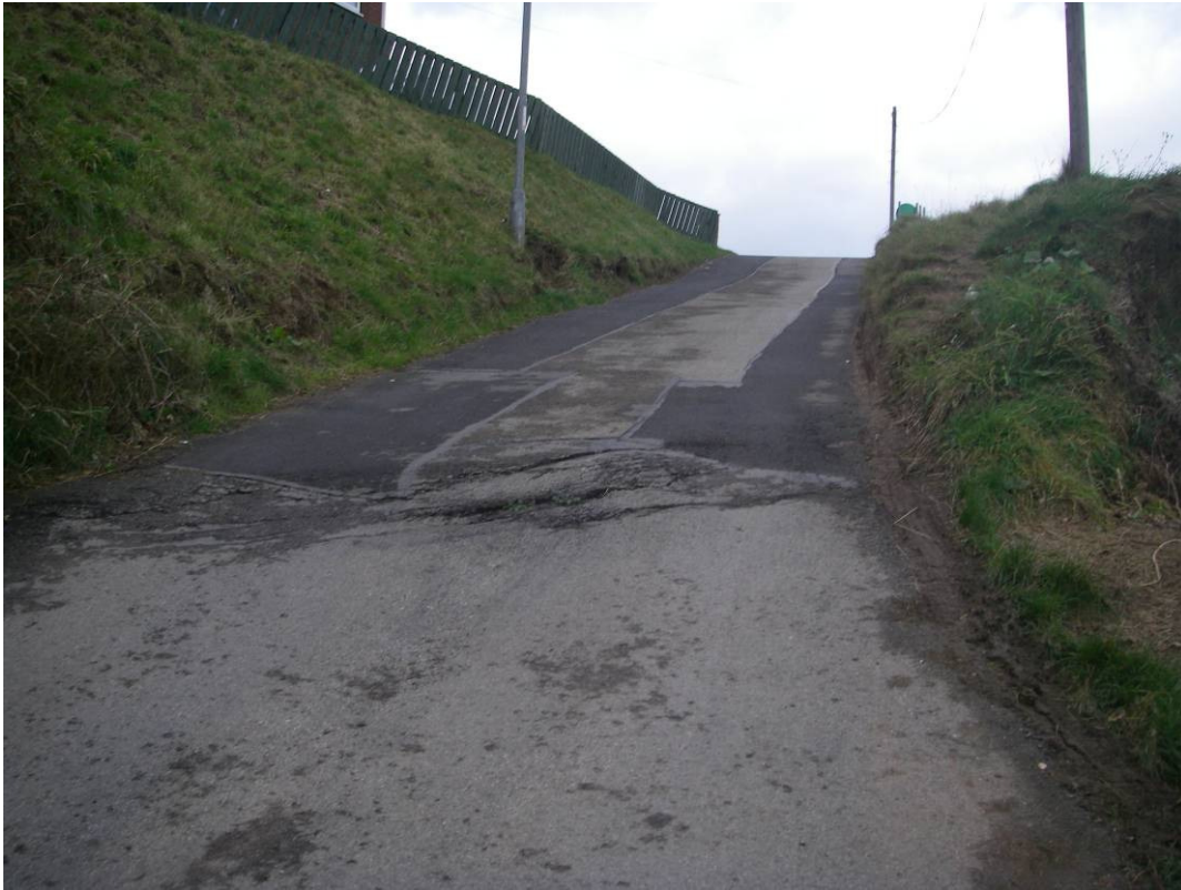
Plate 55 Site view of tension cracks in access road into Flat Cliffs.
