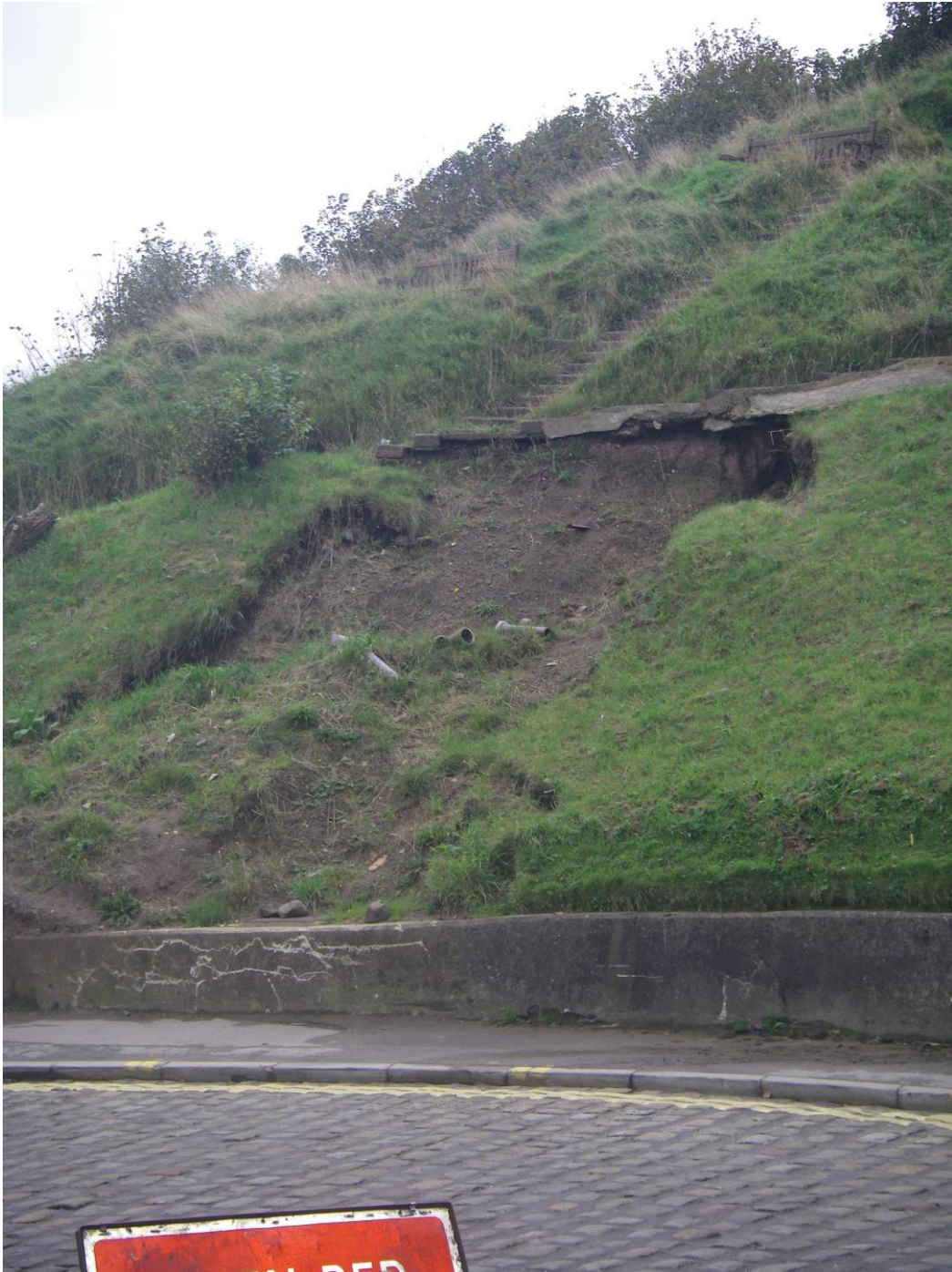
Plate 42. Site view of Crescent Hill showing lower slope failure.
